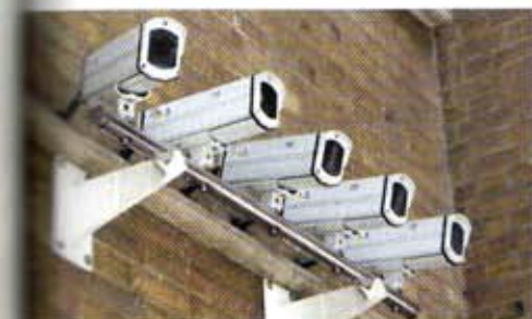
a CCTV camera
